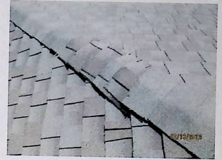
Improperly repaired ridge.
