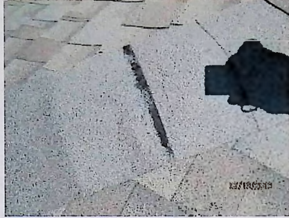
Improperly repaired ridge.
