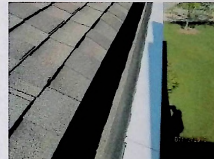
Evidence of moderate to severe hail damage at rain gutter
