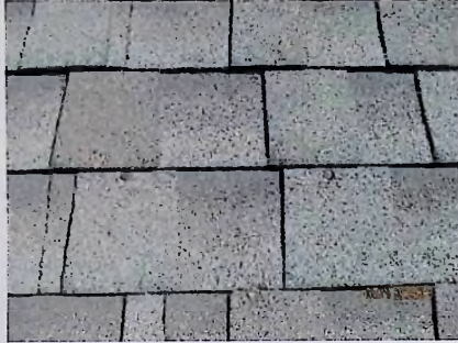
Improper repair and exposed nails.
