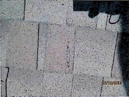
Evidence of moderate to severe hail damage.
