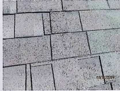
Improper repair and exposed nails.
