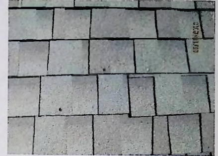
Improper repair and exposed nails.
