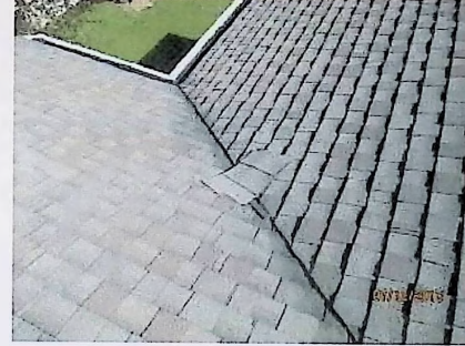
Detached ridge material at valley.
