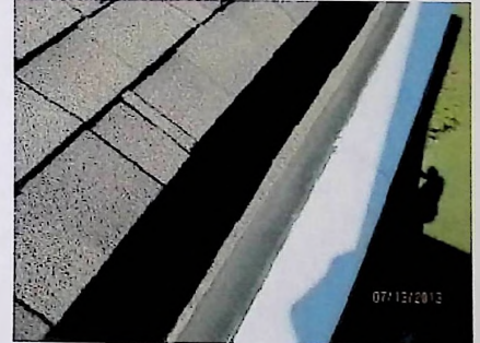
Evidence of moderate to severe hail damage at rain gutters.
