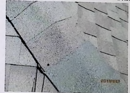
Exposed nails at ridge.
