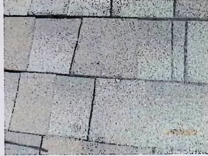
Improper repair and exposed nails.
