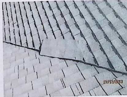
Detached ridge material at valley.
