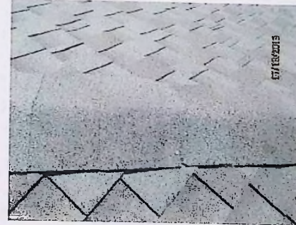
Damaged ridge and exposed nails.
