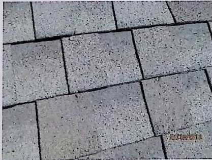
Improper repair and exposed nails.
