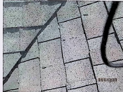
Evidence of moderate to severe hail damage.
